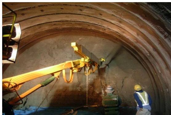
TBM Tunnel Linings
